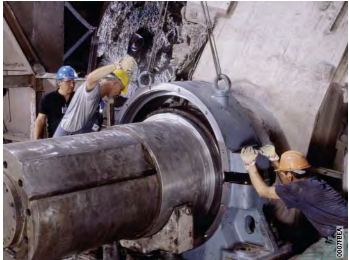
Figure 3 Mounting service on a converter
